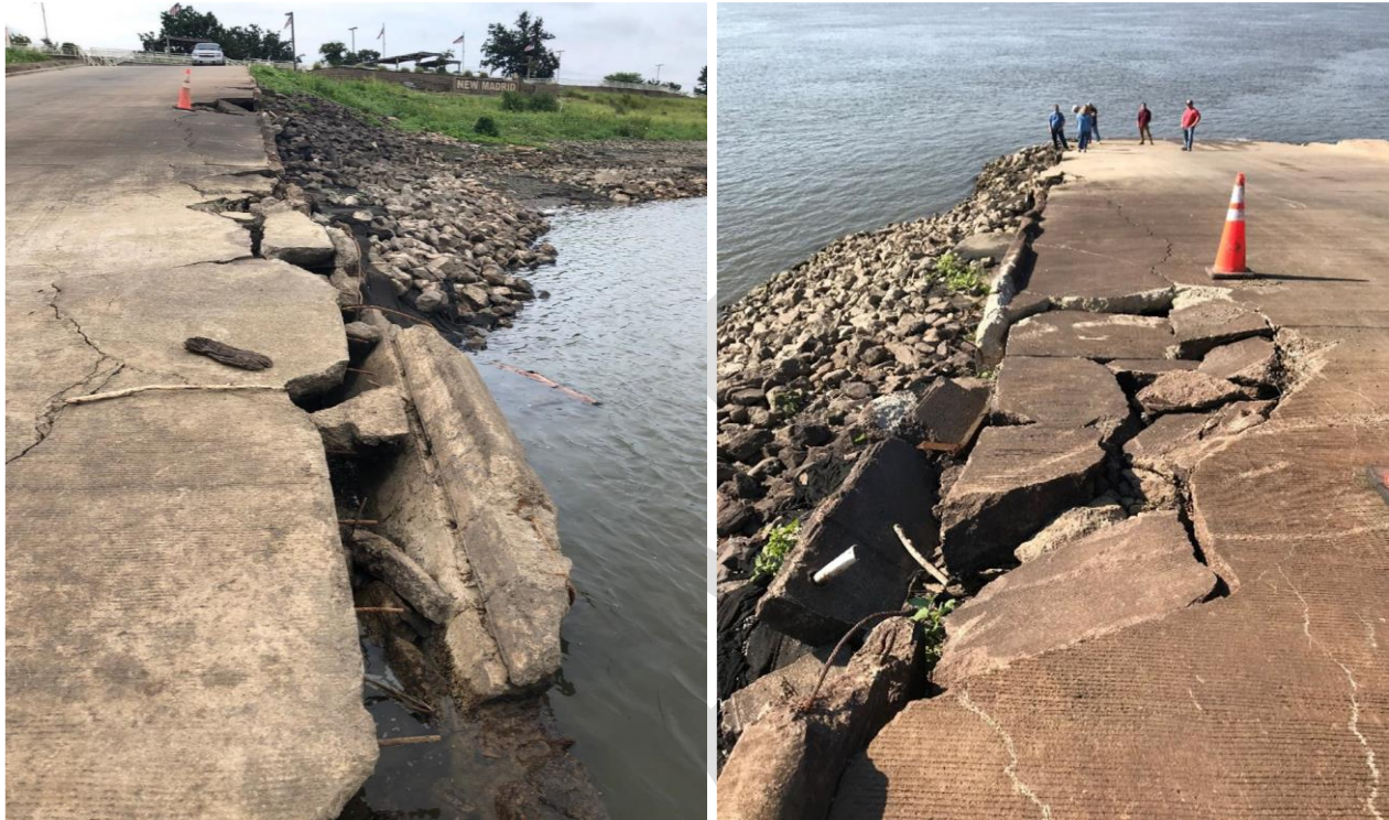
Figures 2 and 3: Concrete damage and scour conditions at the New Madrid boat ramp, New Madrid County, Missouri.
