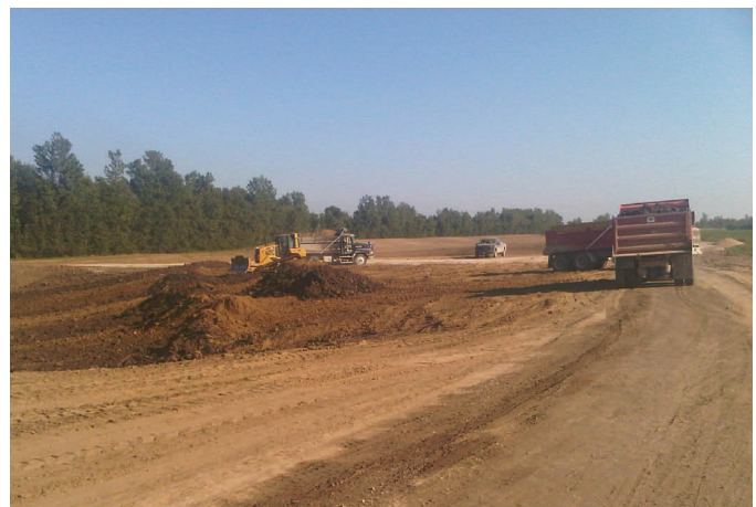
Placing clay into the third of five scour holes today. Crews previously filled the holes to the water table with sand, and are now placing clay in the hole to provide a stable base for the levee and to resist seepage.
