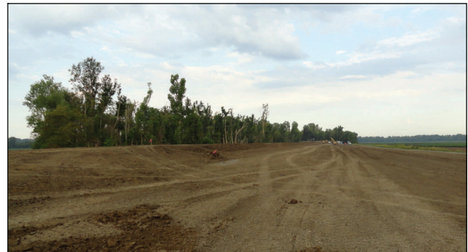
Crews finish a 2,000-foot levee segment at the western end of the lower crevasse.
