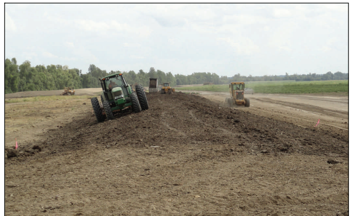
Constructing the realignment at the upper crevasse. Crews spread and compacted clay into the levee today to repair the segment to the interim elevation.
