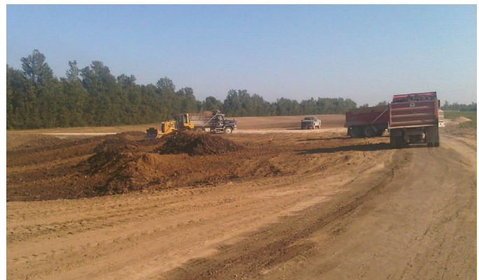
Placing clay into the third of five scour holes Monday. Crews previously filled the holes to the water table with sand, and are now placing clay in the hole to provide a stable base for the levee and to resist seepage.
