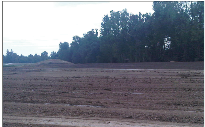
A nearly-complete levee segment at the upper crevasse. Later this week, quality assurance inspectors will verify that this segment complies with our requirements for interim elevation and cross section.
