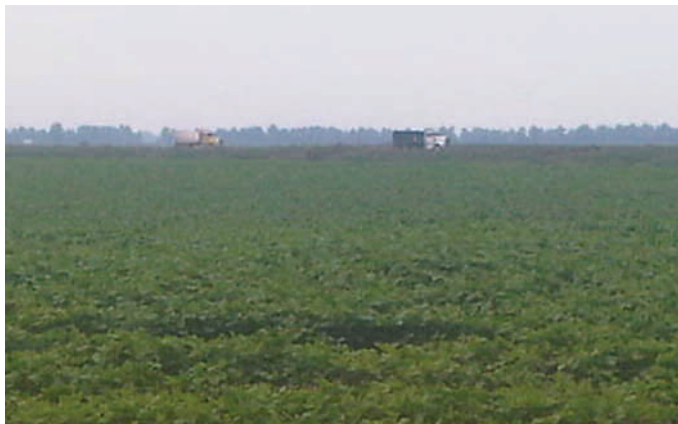
Dump trucks leave the site after delivering sand at the upper crevasse. More than 84,350 tons of sand have been delivered to date.
