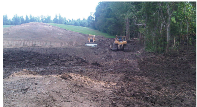
A crew places clay over the first scour hole. The hole had been filled with sand and is being capped with clay to prevent seepage.
