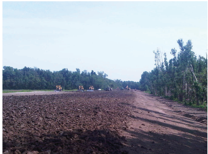
The levee takes shape at the lower crevasse. The river-side slope is now clearly visible.
