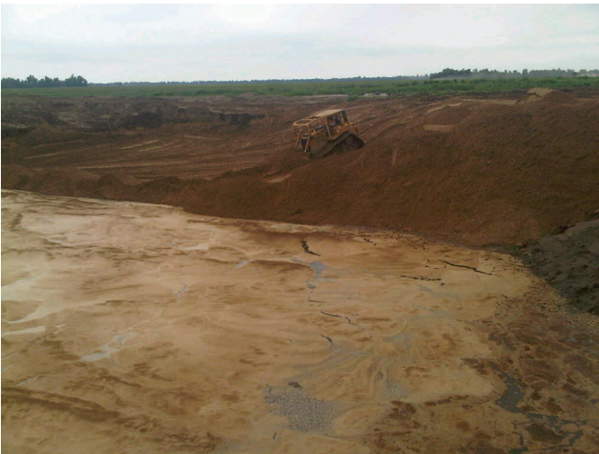
Sand is used to fill a scour hole at the upper crevasse. Clay will be placed over the sand, capping the scour hole and preventing seepage.
