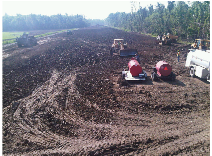
A Vicksburg-based crew prepares the ground at the lower crevasse. The excess water in the soil must be removed before it can be used in the levee.
