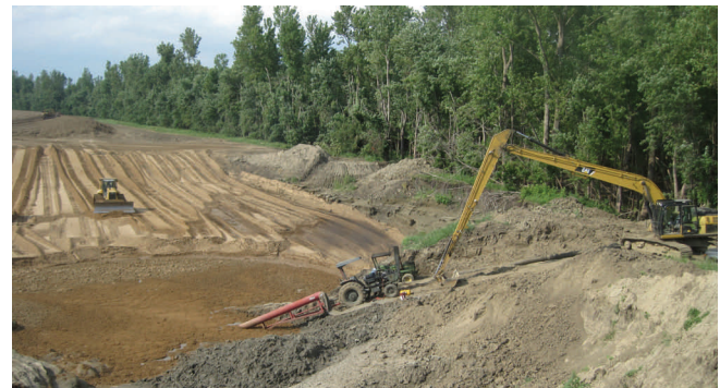
Crews fill a scour hole with sand at the upper crevasse. Clay will be placed over the sand to prevent seepage and bring the hole to level grade.
