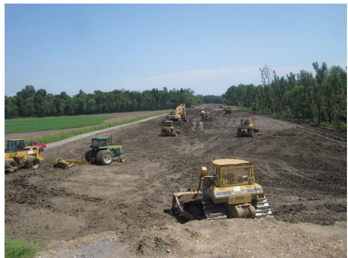
A Vicksburg-based crew removes excess water in the soil at the lower crevasse. Once at the proper moisture content, the material will be compacted into the levee.
