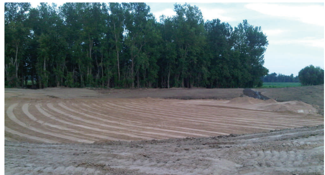
A third scour hole is nearly filled with sand at the upper crevasse. Clay embankment will be placed over the sand up to level grade to prevent seepage.
