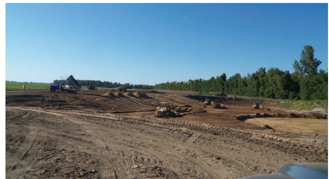
Filling the fourth of five scour holes at the upper crevasse. This hole has been filled 67 percent of the required depth of sand and will be capped with clay.
