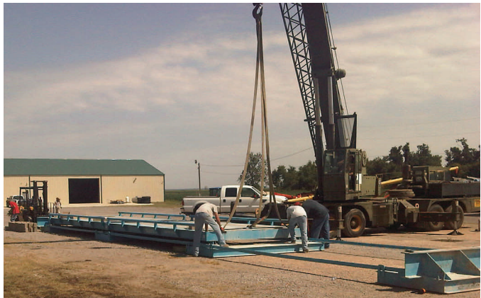
A contractor sets up temporary scales in preparation for clay hauling Thursday. Delivery of clay embankment began Friday.
