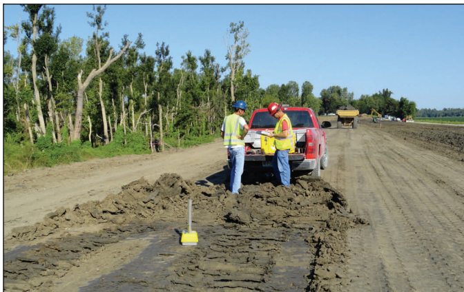
A crew reads the results of a compaction test at the lower crevasse. Seven tests were conducted Sunday and all showed passing results. The tests ensure the levee is being built to the design specifications.
