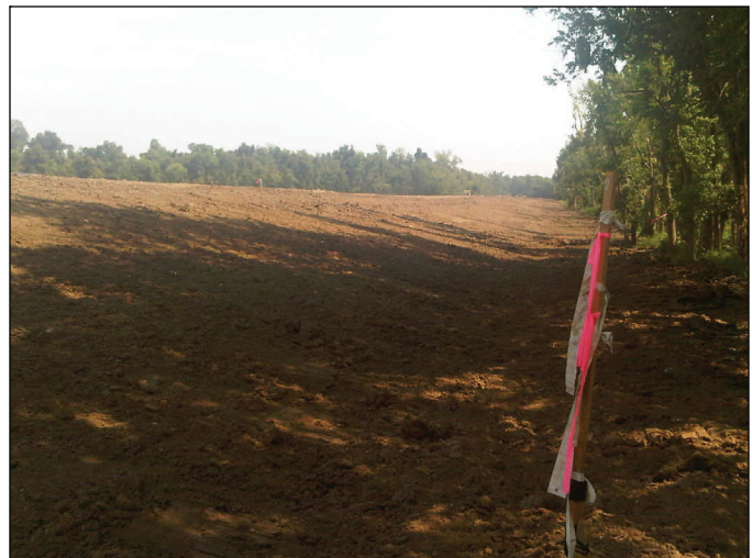
The levee at the western end of the lower crevasse is within three feet from the interim protection elevation.
