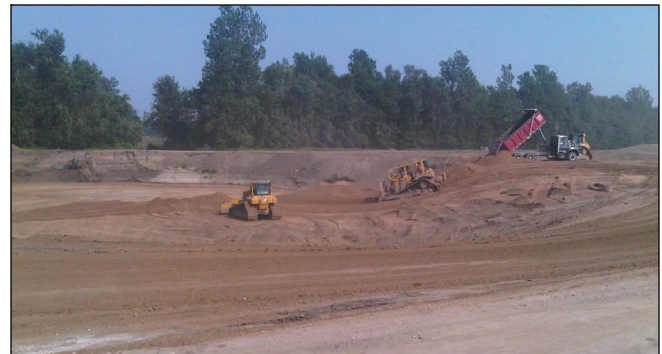
Filling the final scour hole with sand. Clay will be used later to bring the hole back up to level grade and prevent seepage.
