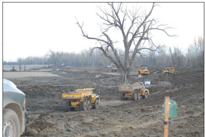
Crews reconstruct levee at the center crevasse Dec. 3 to close an 800-foot gap here.
