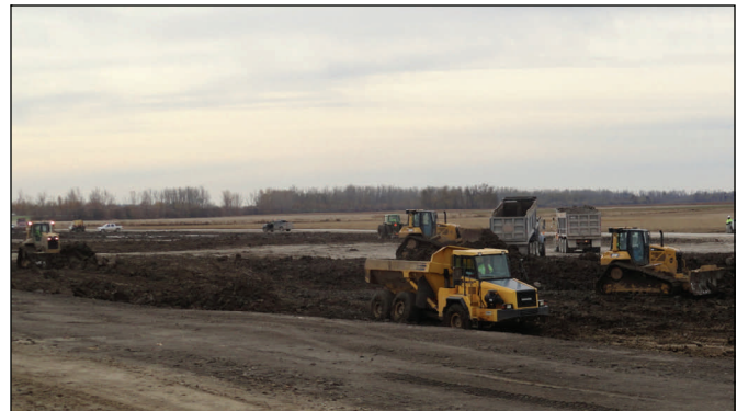
Crews spread clay landside of the levee at the upper crevasse Saturday.
