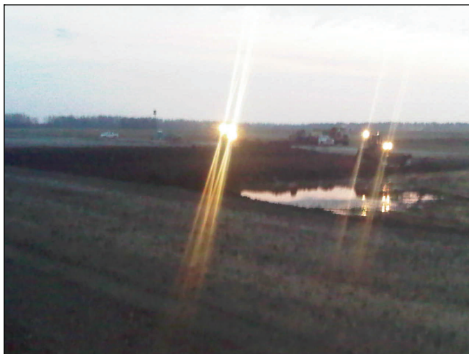
Two bulldozer operators spread clay at dusk Monday at the upper crevasse.
