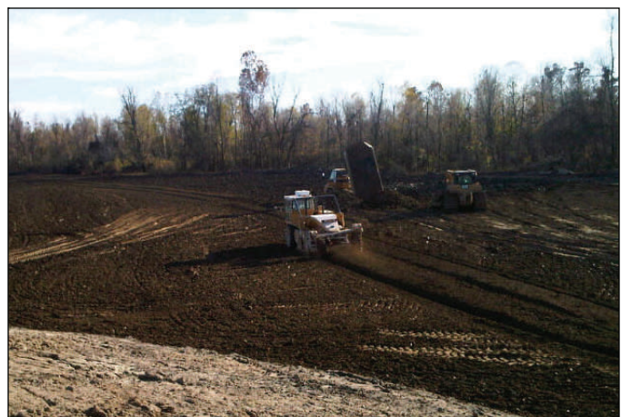
Crews deliver and spread clay Friday at the center crevasse to begin levee reconstruction.
