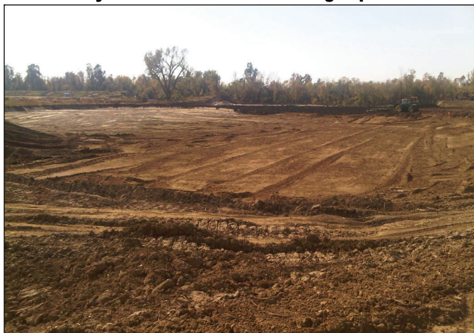
The scour hole at the center crevasse is filled with sand. Dredging ended Monday morning.
