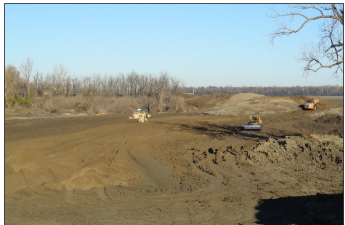
Crews deliver and spread clay Nov. 18 at the center crevasse to begin levee construction.
