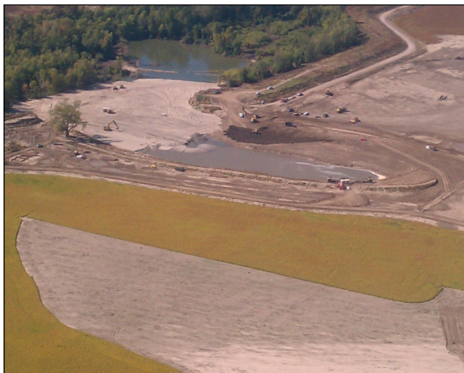
The center crevasse scour hole as seen from the air Oct. 25 during dredging. The area to the right of the levee was filled in after this photo was taken. (Photo by Brad Hahn, courtesy of Great Lakes Dredge & Dock Company)
