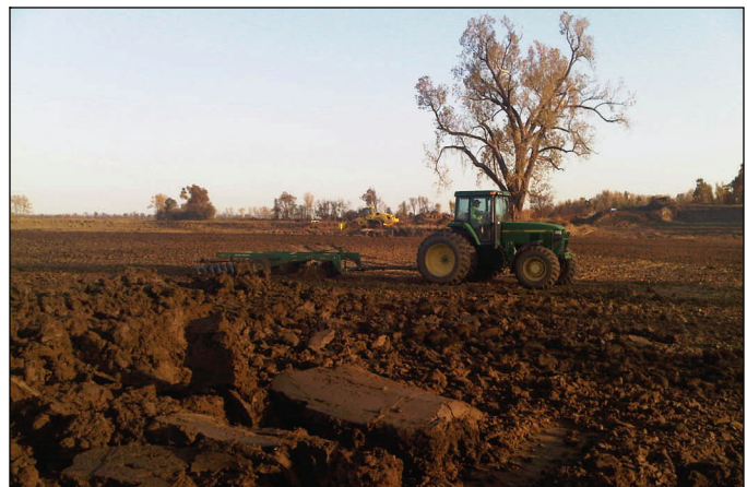
Crews disk and compact clay after it is placed in the scour hole at the center crevasse Monday.
