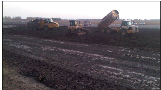
Crews spread clay landside of the levee at the upper crevasse Monday.
