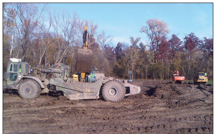
Crews load clay at a newly-acquired borrow site Monday. The clay is bound for the scour hole at the center crevasse.
