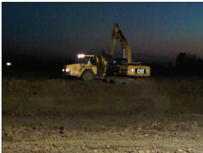
An excavator operator loads an off-road dump truck Monday night with clay that will fill the land-side berm. Each off-road truck can carry up to 25 tons of clay. The District began night operations Saturday.
