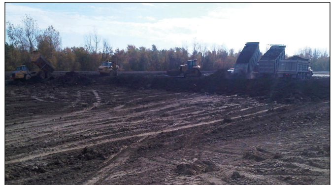
Crews spread clay landside of the levee at the upper crevasse Tuesday.
