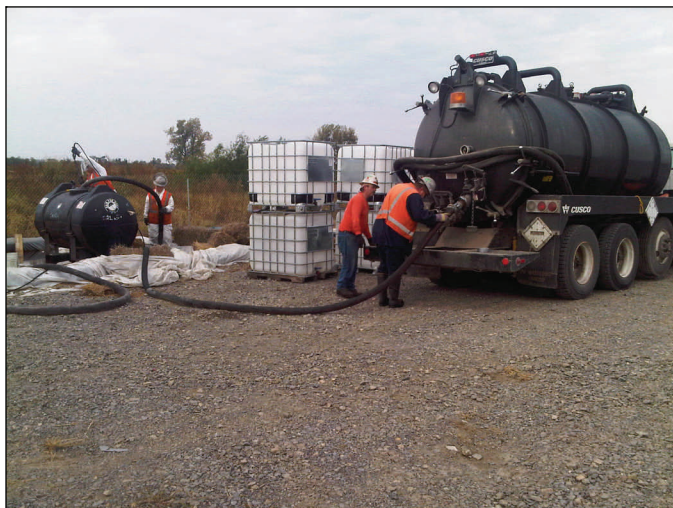
A contractor at the upper crevasse transfers desensitized blasting agent from the storage containers (at left) to USDOT-authorized shipping containers (at center) Wednesday. Removal will begin later this week.
