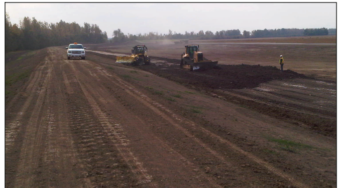
A bulldozer operator spreads clay landside of the levee at the upper crevasse Wednesday.
