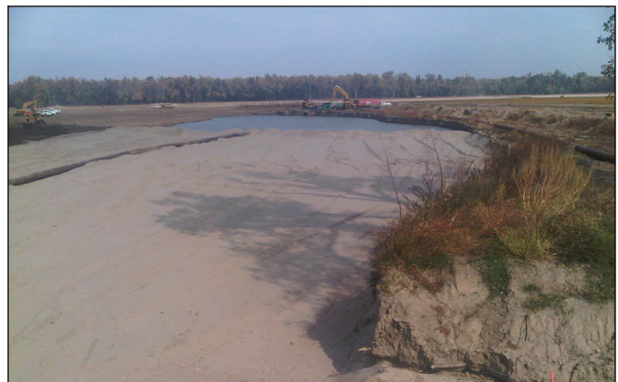
The dredge contractor pumps sand into the scour hole at the center crevasse Wednesday.
