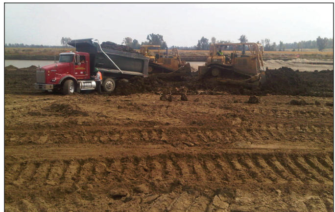
Clay is delivered to the center crevasse Wednesday to cover the dredge sand that was placed in the scour hole. This clay will form the foundation of the levee and serve as a landside seepage barrier.
