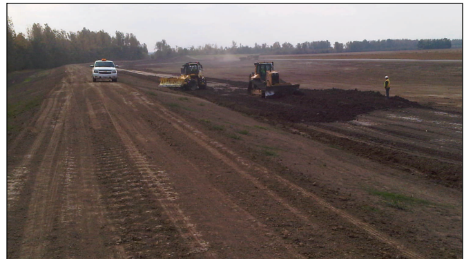
A bulldozer operator spreads clay landside of the levee at the upper crevasse Oct. 26.
