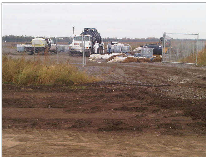
A contractor at the upper crevasse transfers desensitized blasting agent into USDOT-authorized shipping containers (at left) Oct. 28.
