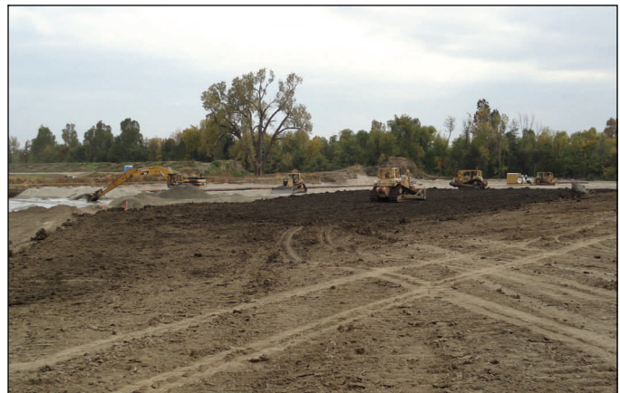
Clay is spread at the center crevasse Oct. 27 to cover the dredge sand that was placed in the scour hole. This clay will form the foundation of the levee and serve as a landside seepage barrier.
