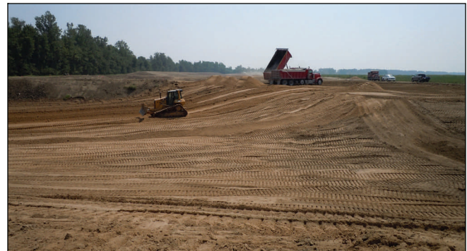
Filling the final scour hole with sand at the upper crevasse near Birds Point. A total of 132,740 tons of sand were delivered for the contract.
