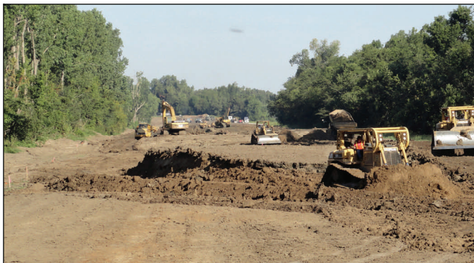
A flurry of activity at the lower crevasse. The crew is preparing the levee foundation and embankment material at the eastern end in preparation for repairs here.
