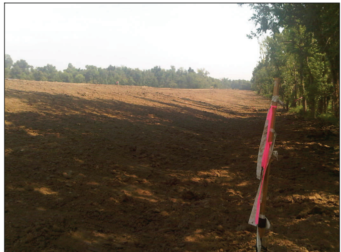
The levee at the western end of the lower crevasse is now within one foot of the interim protection elevation.
