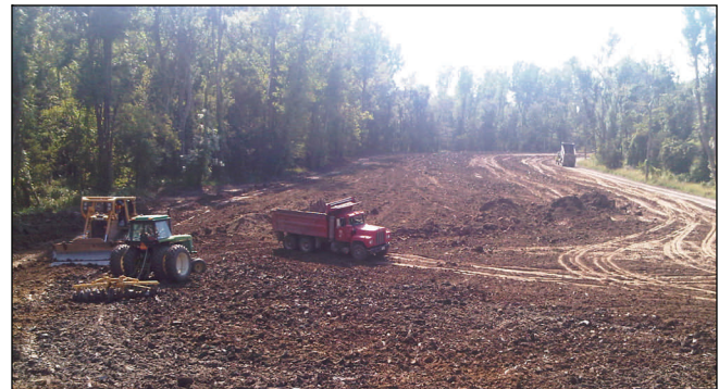
Work at the lower crevasse resumed today after rain delays. Crews are processing material to remove excess water before placing the clay into the levee.
