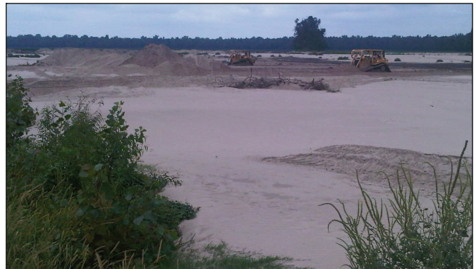
Crews at the center crevasse harvest sand from the surrounding fields Tuesday. The sand is being transported to fill the single large scour hole here.
