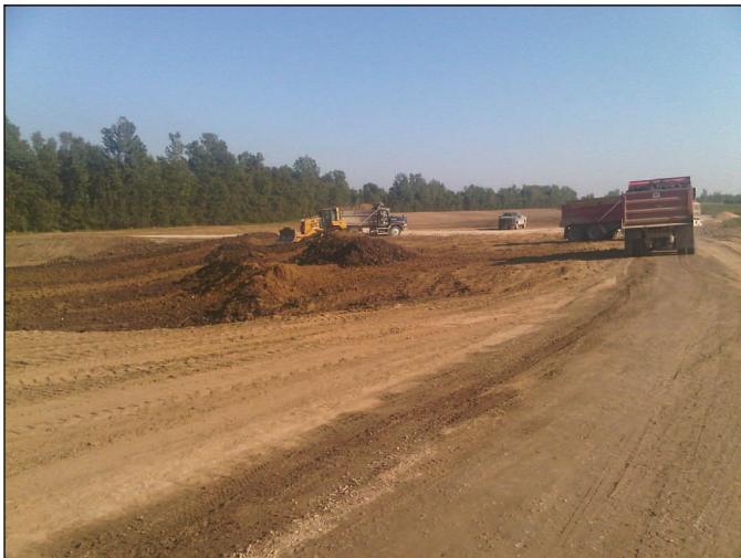
Placing clay into the third of five scour holes Sept. 12. Crews previously filled the hole to the water table with sand, and are now placing clay in the hole to provide a stable base for the levee and to resist seepage.
