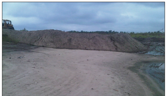
Sand from surrounding fields is being used to fill the scour hole at the center crevasse. As of Tuesday, crews had placed a sand shelf approx. 50 feet long by 75 feet wide in the scour hole.
