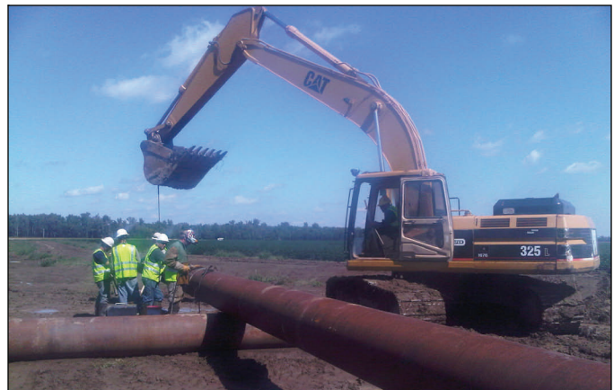
A welder for the dredge contractor joins pipe Monday at the center crevasse. When fully assembled, the pipeline will transport river sand more than a mile to fill the scour hole.
