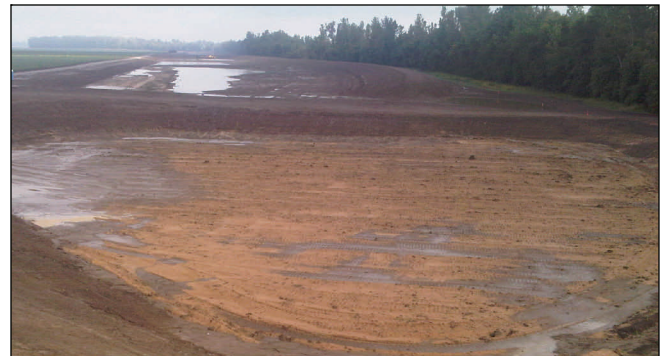
Monday morning was wet and muddy at the upper crevasse. Afternoon sun helped to dry the ground, but not yet enough to support heavy equipment.
