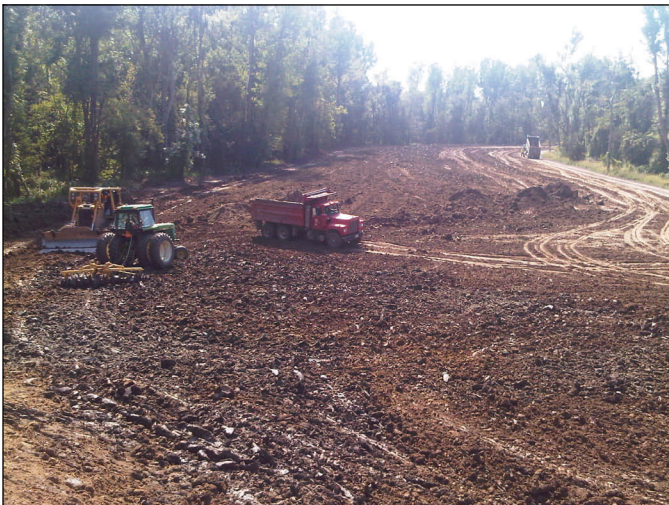
A Vicksburg crew processes material Sept. 21 at the lower crevasse to remove excess water. The soil here is poorly drained and extra effort is required to reduce the moisture content to a workable level. The crew will resume processing material Tuesday.
