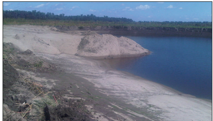
Sand begins to fill the scour hole at the center crevasse Monday. The sand was harvested from the surrounding fields and hauled to the scour hole.
