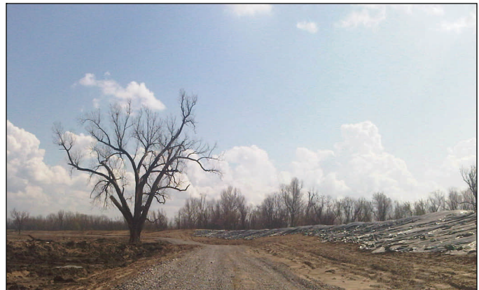
The repair team completed the center crevasse access road in late February. The road provides all-weather access to the levee. March 15 photo.
