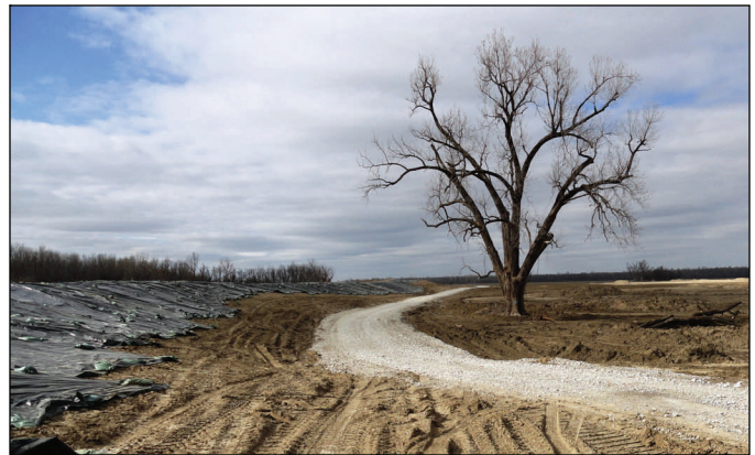
The repair team completed the center crevasse access road in late February. The road provides all-weather access to the levee. March 1 photo.
