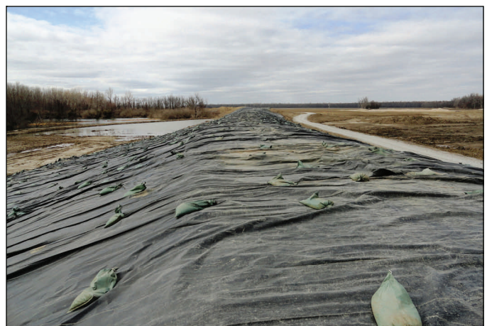
A March 1 view of the repaired levee at the center crevasse. The access road is visible at right.
