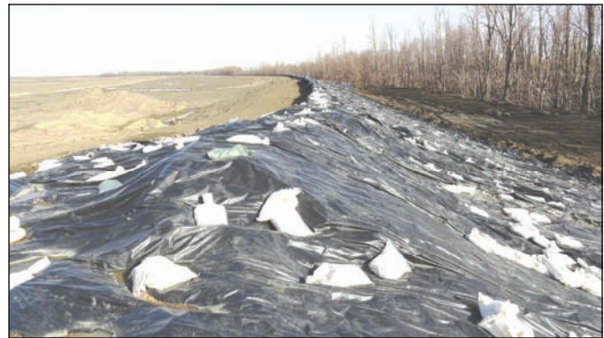
Plastic sheeting to protect the levee and HESCO barriers is shown in this March 1 view.
