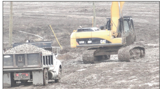
The District's repair team places rock at the center crevasse Wednesday to stabilize the roadway.
