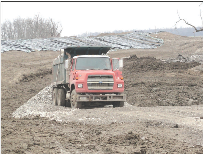
The team performs road maintenance at the center crevasse Feb. 9. Here, the team places rock to stabilize the eastern access road.
