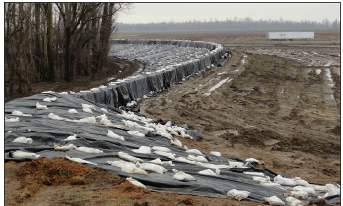
The repair team completed repairs to the plastic at the upper crevasse Feb. 2. The team also added additional sandbags to better hold the plastic in place.
