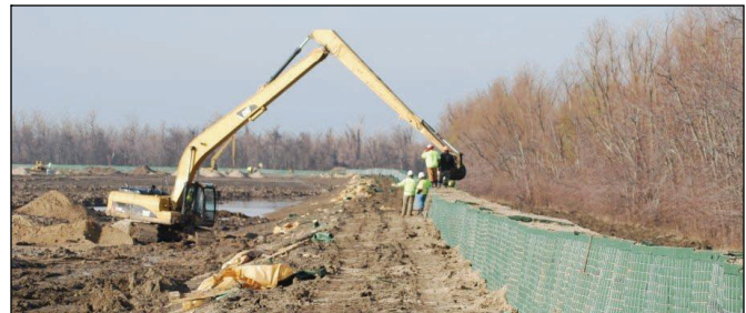
A crew fills HESCO barriers at the upper crevasse Dec. 11. The barriers are a temporary measure to raise the level of protection at Birds Point from 51 to 55 feet on the Cairo gage. Permanent repairs to the levee will resume after spring highwater recedes.
