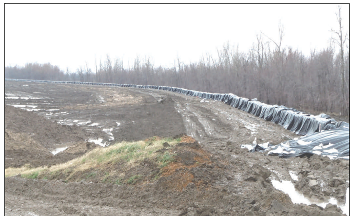
HESCO barriers span the length of the upper crevasse Dec. 15. The plastic sheeting protects against erosion and provides a water-resistant barrier over the HESCOs.
