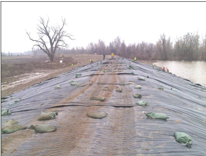
Crews cover the newly-constructed levee segment at the center crevasse with heavy plastic sheeting Dec. 6. The plastic sheeting will help protect the levee against erosion caused by wave action and rainfall. This view looks east along the levee.
