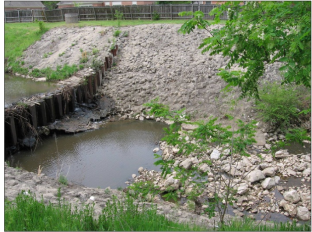
Weir and bank after reconstruction. Note erosion occurring at edge of the existing concrete apron.
