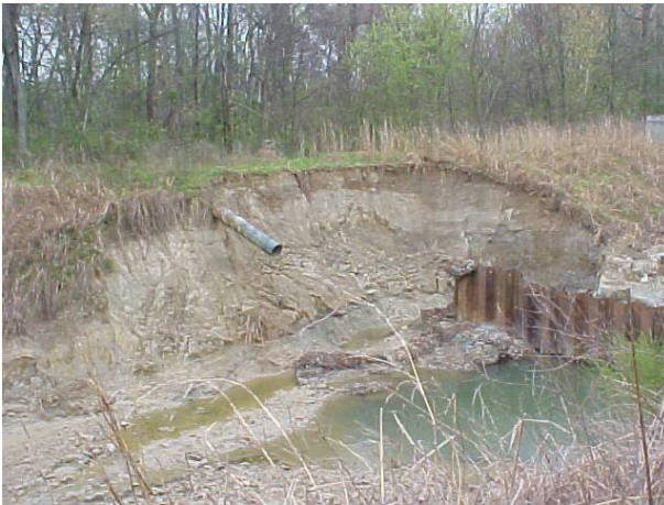
Previous bank failure at weir location. Storm main is visible on the right edge of the picture.
