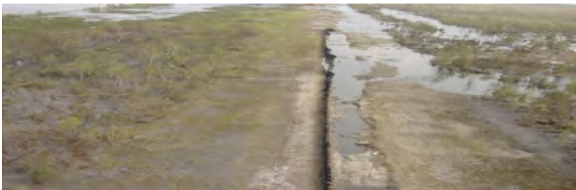
Figure 13. Levee Damage after Hurricane Katrina
